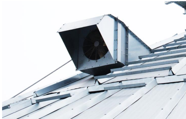
Figure 14: Silo Roof Exhaust Fan
